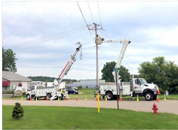
Made-for-TV moment: In July, crews from Jefferson Utilities set up this work zone to allow MEUW to capture video footage for a promotional spot that will air on Wisconsin Public Television this fall.
